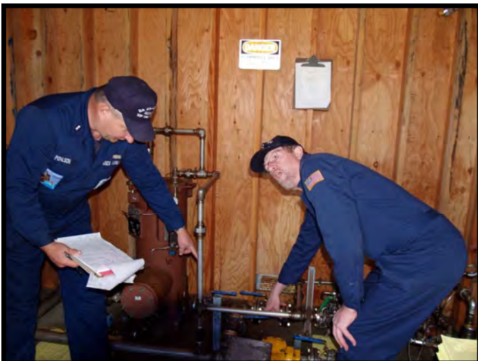
Auxiliarists Doug Pohlson and Ken Reynoldson check the valve system during training on the fuel system.
