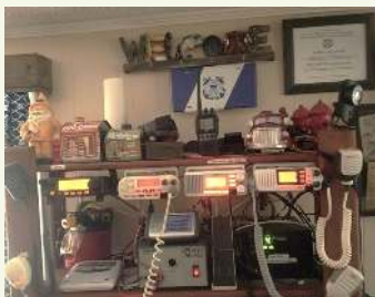
Houghton Lake Fixed Radio Facility
