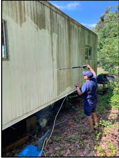
Larry Cole (FC 25) cleaning the Flotilla 25 Operations Center in prep for a much- needed paint job. Photo by Steve Siske.
