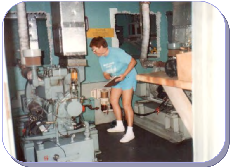
Right, Dolores Spain taking readings on the generator's gauge that keeps the lighthouse operational. Photo by J. Spain
